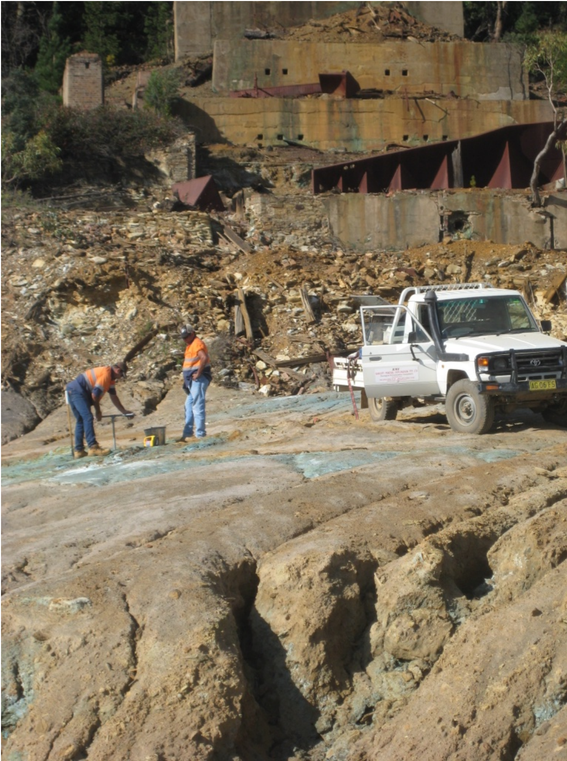
Figure 2 - The Tailings Sand Being Sampled With an Auger Drill With The Old Treatment Plant Foundations In The Background
